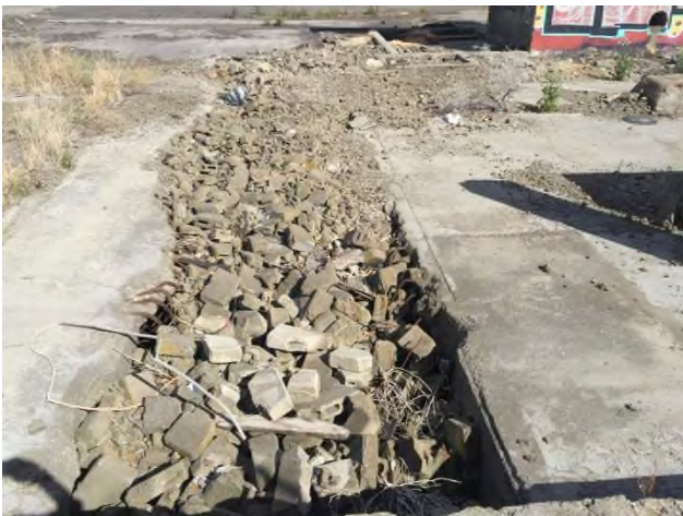
Plate 6: Narrow underground 'passage', filled with rubble on the western side of the building slab
