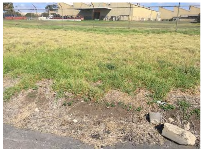
Plate 9: Edge of access roads in south western corner approx. 0.5 m below level of surrounding land
