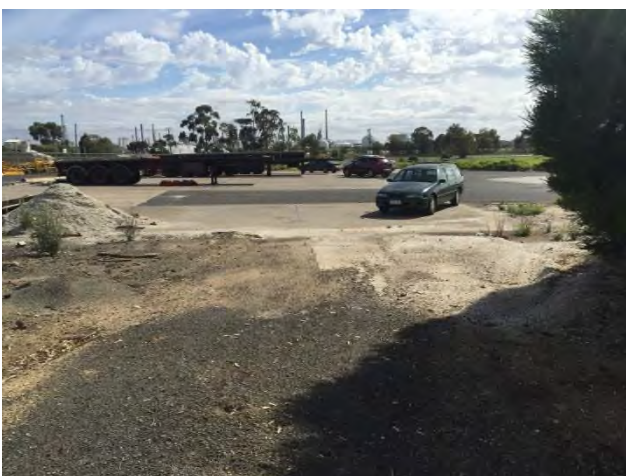
Plate 14: Large concrete apron on the NW side of the former Mill building, looking north
